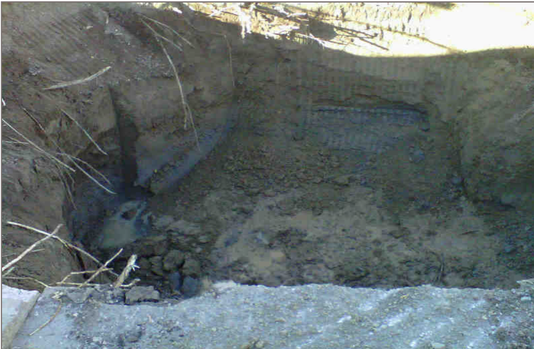
Photo 6: View showing south and west walls and base of excavation. Darker coloured areas are indications of staining.
