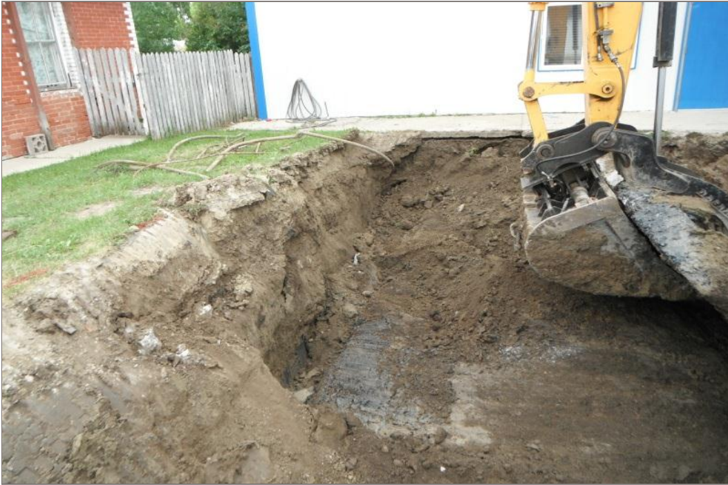
Photo 5: View showing stained soil at an approximate depth of 1.5 mbg.
