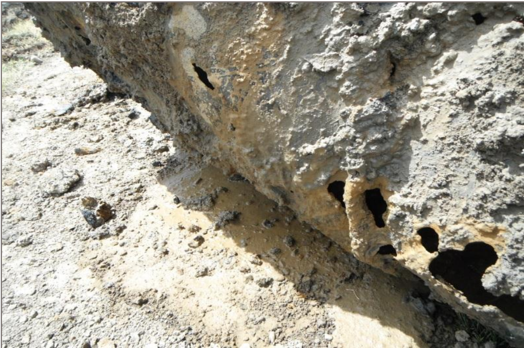
Photo 4: Close up view of UST showing corrosion and holes.
